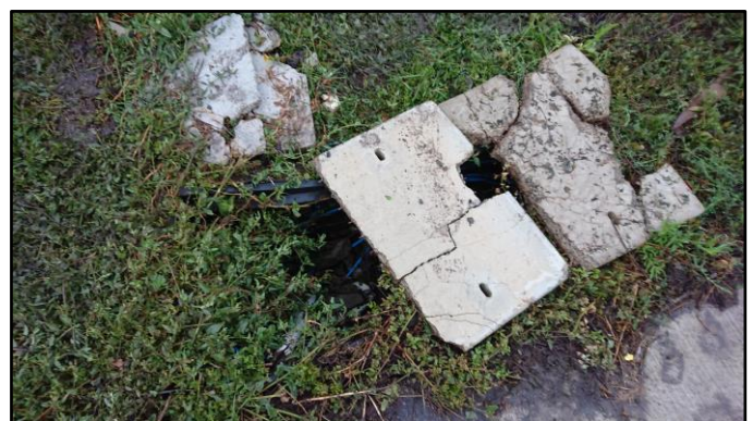
IDENTIFIED - Near miss involving hole on site
